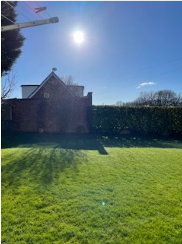
Photo 4: View of the existing gable of No.4 (wall of the garage forming part of the boundary) taken from the rear of No. 2 Lindsay Park
